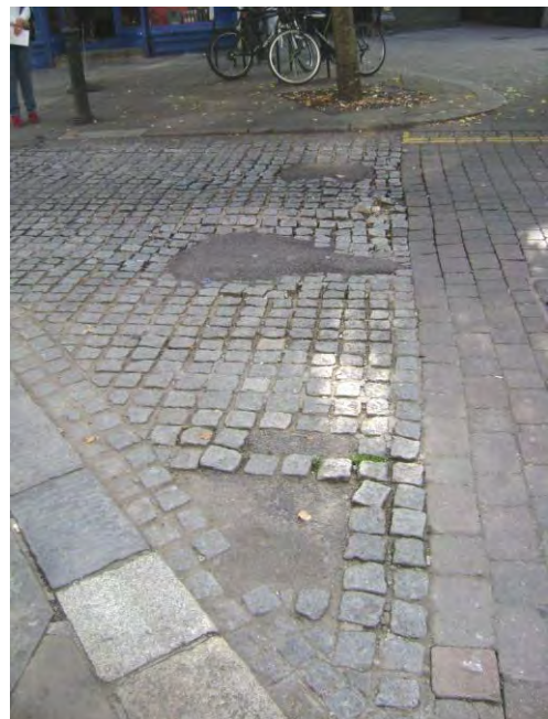
Broken and uneven paving is a hazard to pedestrians
