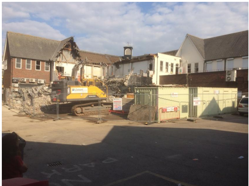
View of demolition works from the car park and the delivery yard. Pictures - Ian Nash
